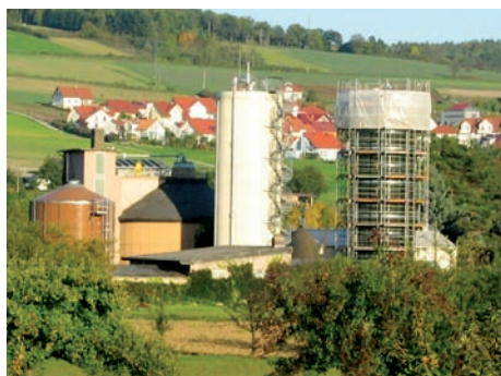
Figure 1: The old sludge digestion plant at Tauberbischofsheim was replaced by a two-stage high-load digestion facility.
