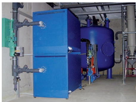
Figure 1: Vacuum plant in the basement of the water house.
